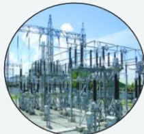
EAF Sub Station
