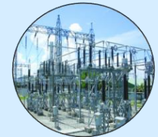
EAF Sub Station
